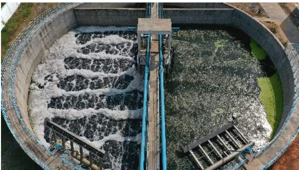
Photo: SBR Basin, 7.6 MLD STP
