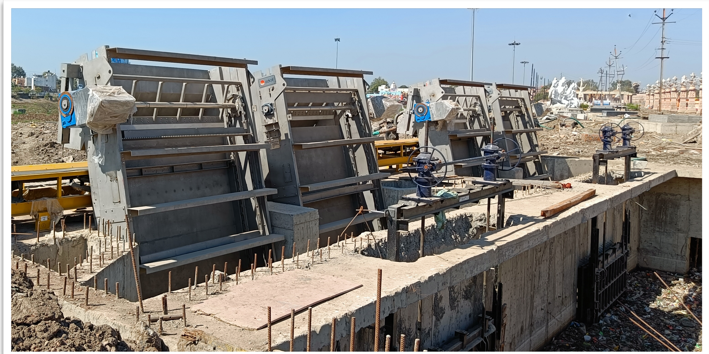
Our installation of 4 Multi-rake Mechanical Screens, 5 Sluice Gates and Conveying System at storm discharge outlet at Rudra Sagar Lake
